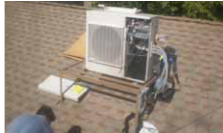
Mini-Split Condensing Unit
